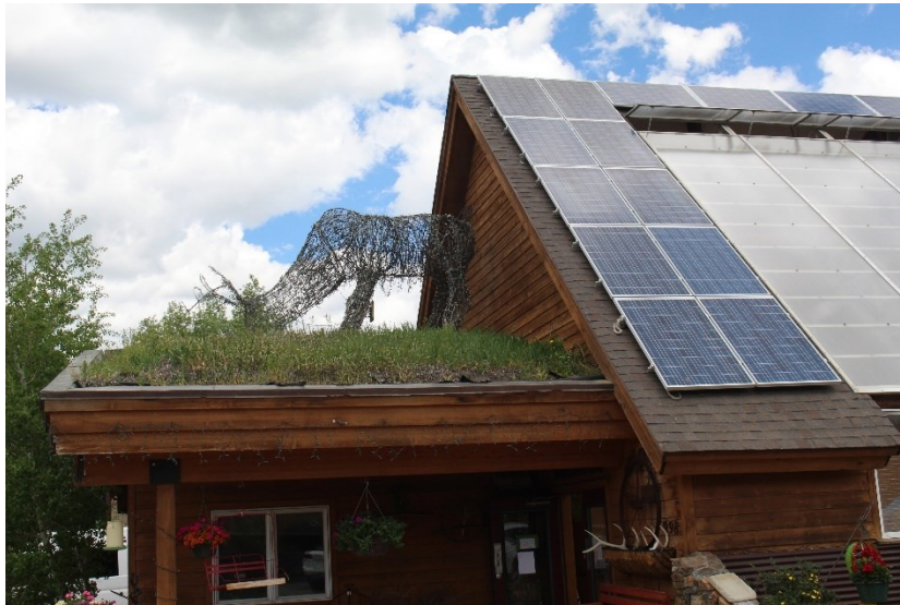
Figure 23. Solar Panels at Alpine Garden Center
