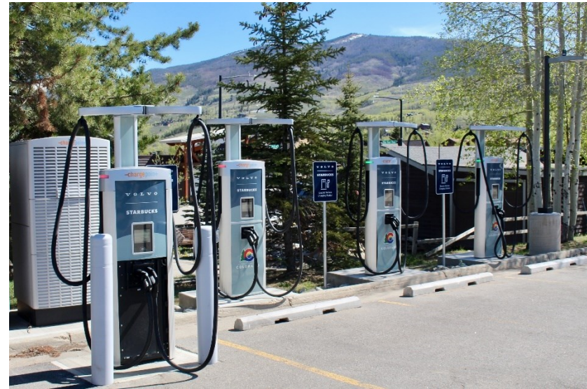
Figure 37. Electric vehicle charging station in the Target parking lot
